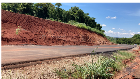
The starting point: an unprotected red-soil cut
