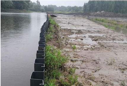
Bank defence: it stops the scour at the toe of the bank
